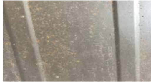
Heavy swarf staining on pre-painted steel.
