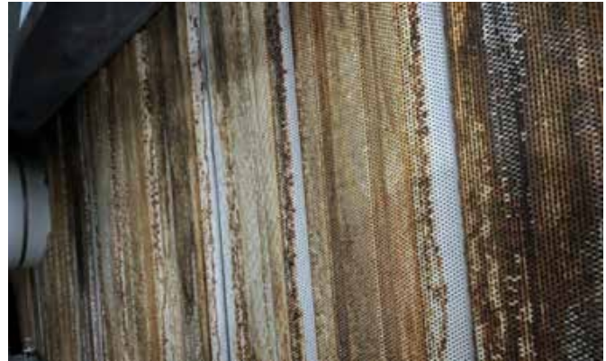
An example of wet stack storage corrosion on a perforated panel
