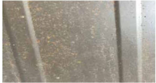
Heavy swarf staining on pre-painted steel.
